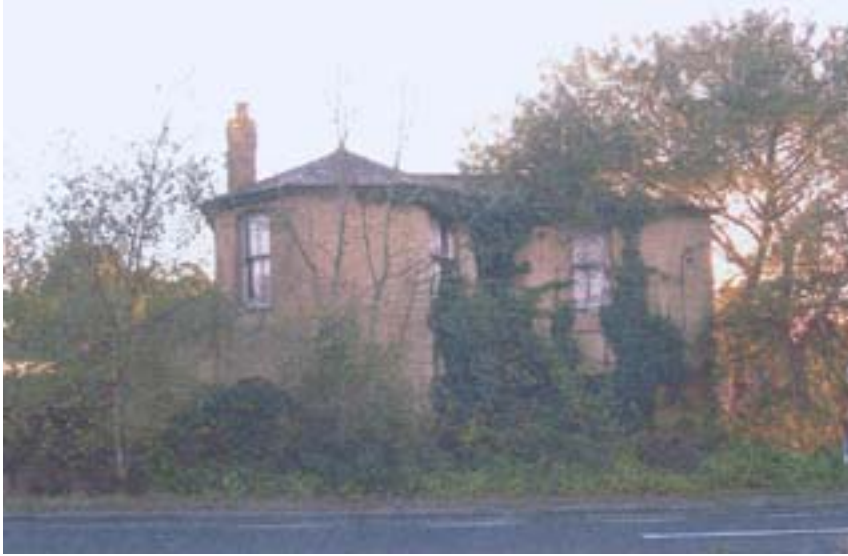
The rapidly deteriorating Park Lane Toll House at Ashton Corner.
